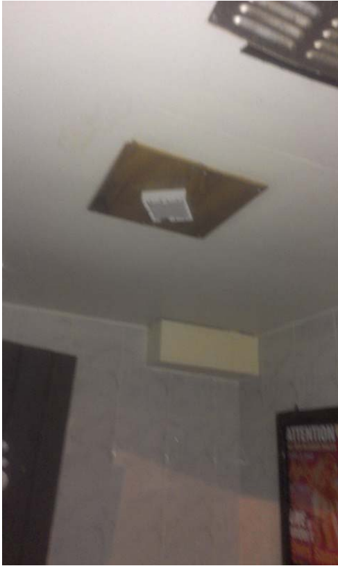
7) Damaged electrical furniture comprising IPX ratings.
