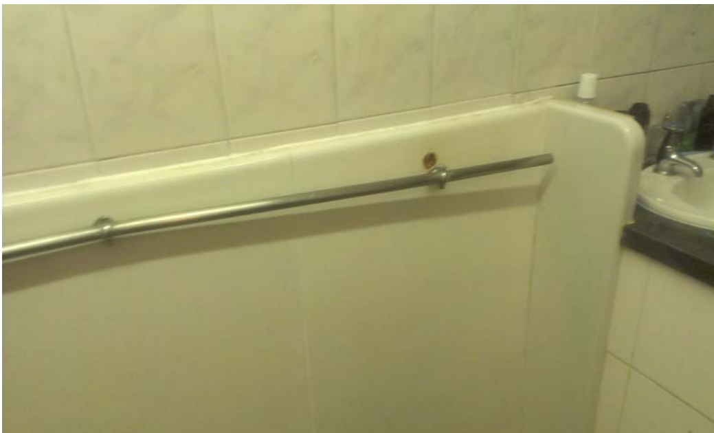
2) Damaged water pipework in toilet area.
