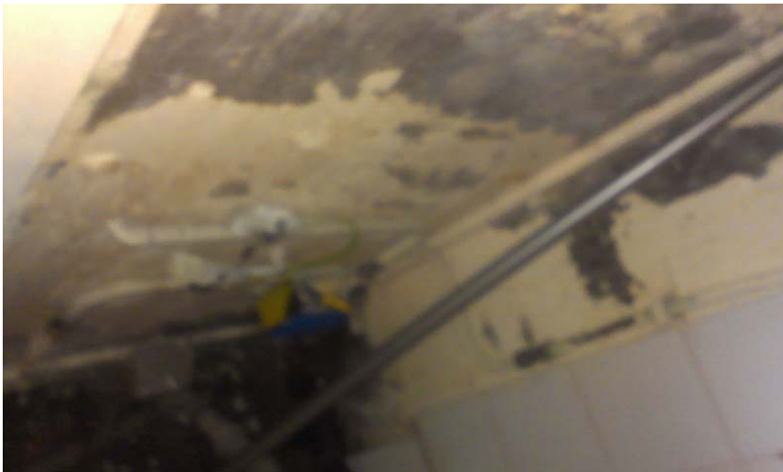
17) Very poorly maintained toilet facilities.
