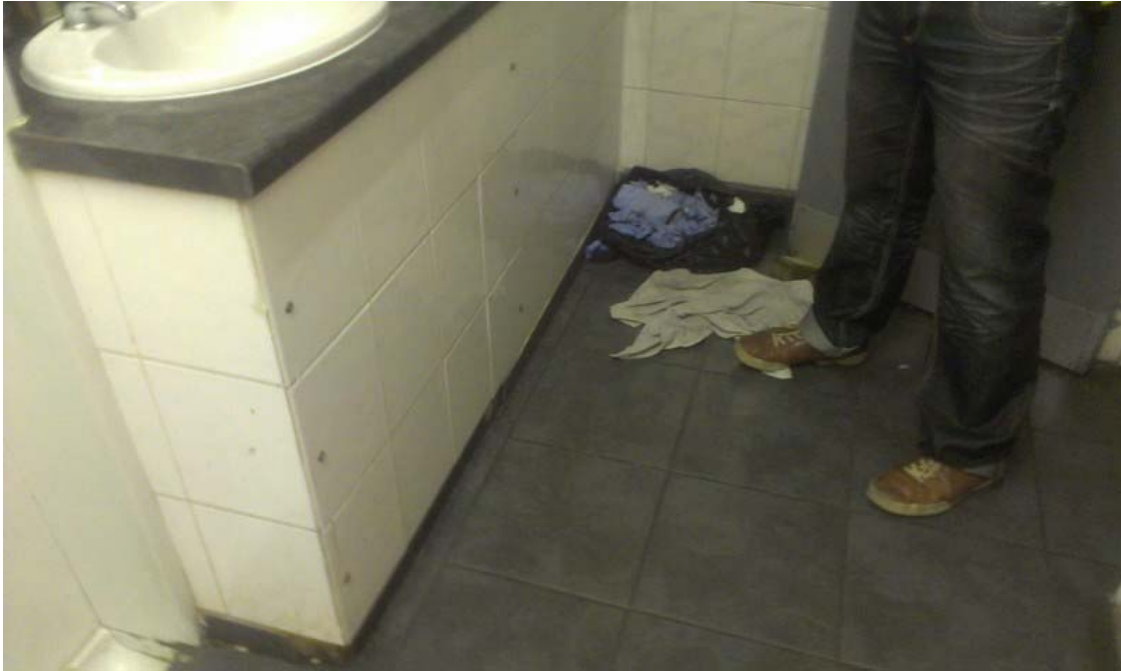
3) Poorly maintained toilet facilities-waste on floor.
